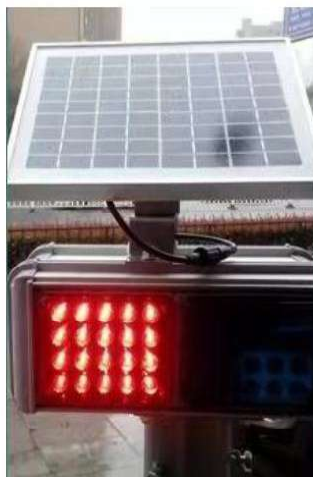
Traffic signal lights
